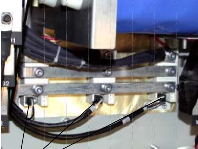
PHOTO 7 SCR Gate Connections VLT 5125-5150
